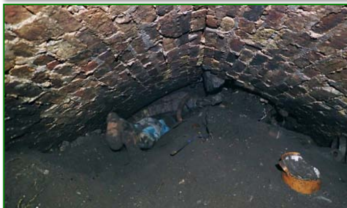
Alan crawling through the ash filled collapse.
