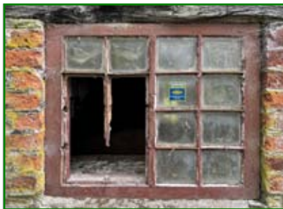
The damaged loco shed window.
