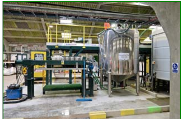
The filter and concentration end of the main plant.
