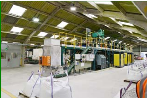
The Lithium pilot plant processing line.
