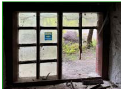
Interior view of the damage.
