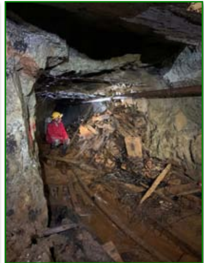
Possible collapsed ore chute in Cligga. (Gareth Rushton)
