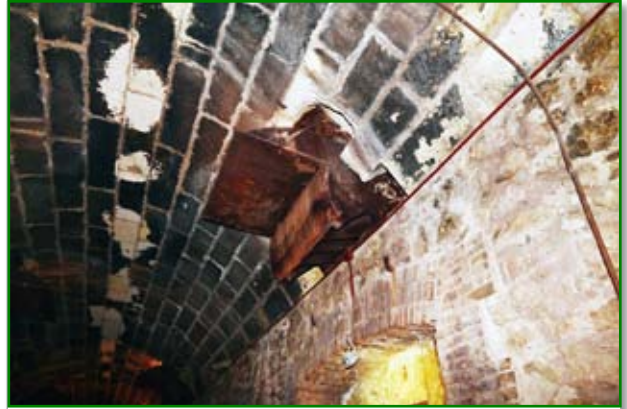
One of the ore chutes in the roof of the railway tunnel.
