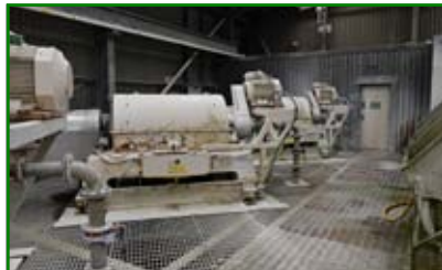
First stage refiners - Supercone separators at Trebal Refiner Site.
