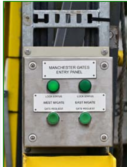
Banksman's controls for the gates at the top of the shaft.
