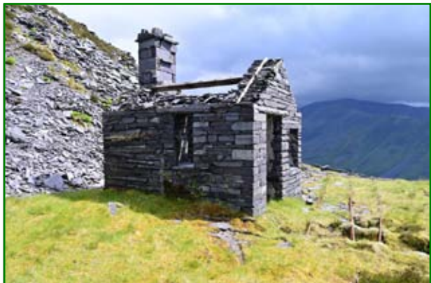
Control cabin on Egypt Level for the C6 Incline.
