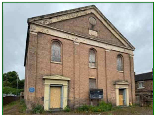
The Fletcher Methodist Chapel is now in a sorry state after being boarded up for over 7 years.
