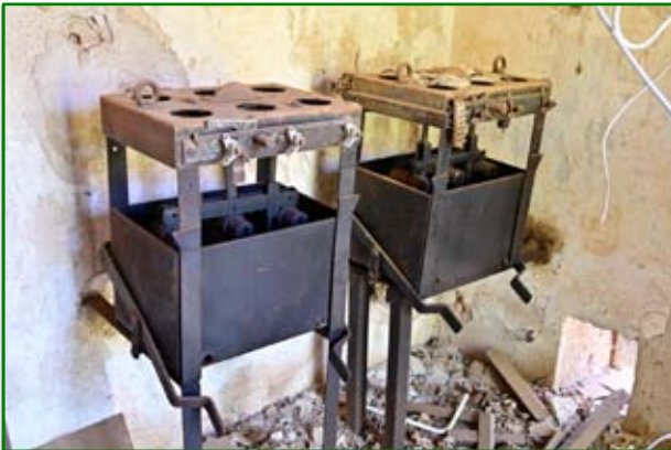
Oil bath switches in the second transformer house.
