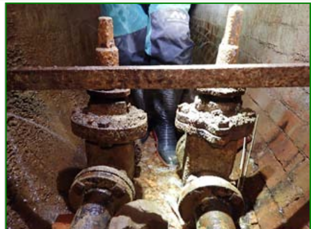
The 2 gate valves near the cistern end of the tunnel. (Vicky Robinson)
