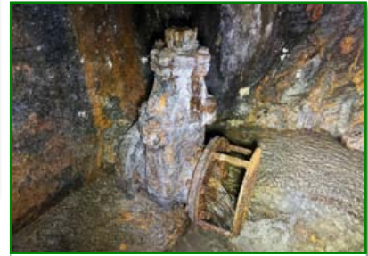
Valve in a dammed level to a quarry used for water. (Kelvin Lake)
