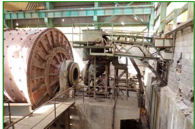
The feed to a ball mill in the Semi-autogenous mill. (Steve Holding)
