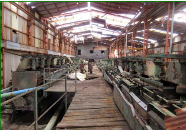
The flotation cells in Lavadero Roberto 2. (Andy Wood)
