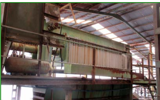
Filter press near the flotation cells, Lavadero Roberto 2. (Andy Wood)
