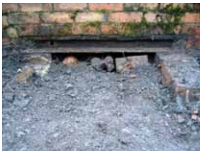
Figure 5, above: Hole in the lintel above the balance beam pit at Billingsley
