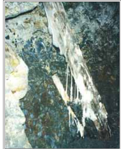
Above: Fungus hanging from timber on the south side of the new concrete section.
