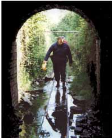
Above: Peter Eggleston in the entrance to "la galerie du Tiefstollen" part of the Chretien Inferieur , with its 1900 rails. [KL]
