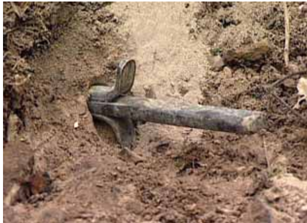
The plug (centre) and feathers (above and below the plug) inserted into the hole, ready to split the rock.
