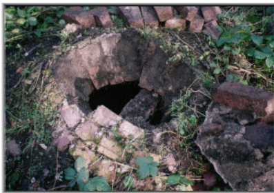
Crown of the broken open shaft cap.
